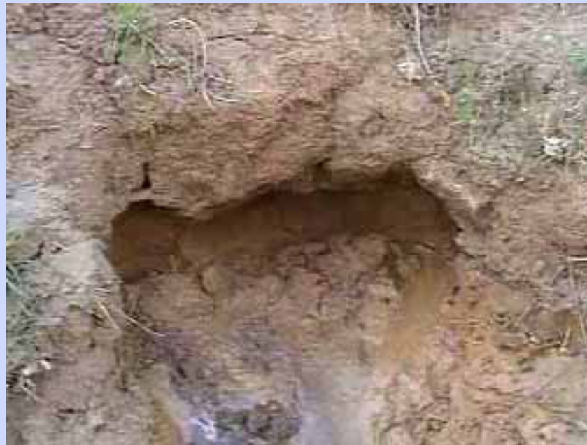
Streambank Seep from Sloughed Deposits
